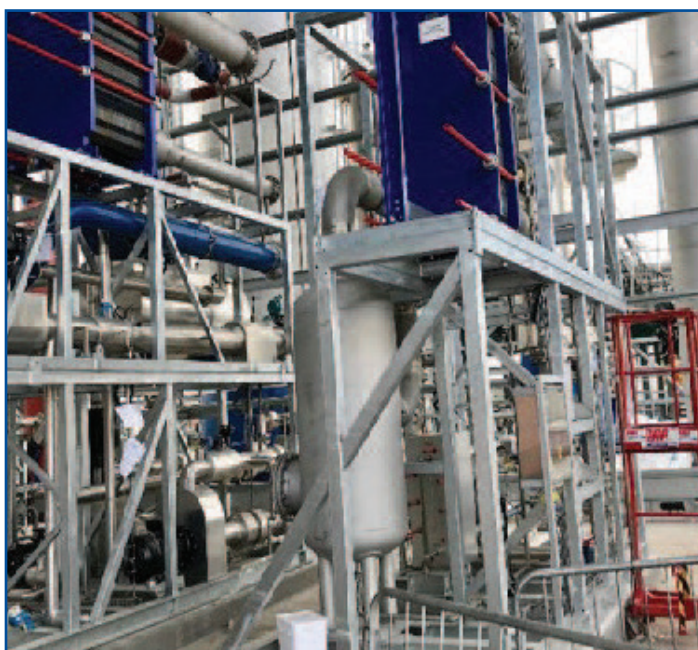
First industrial scale CCU plant in the UK. Image provided by Tata Chemicals Europe.
