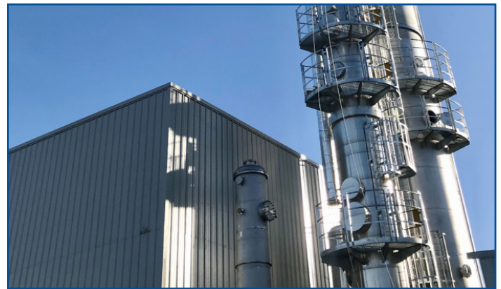
Scrubbing Tower at the TCE CCU plant in the UK. Image provided by Tata Chemicals Europe.
