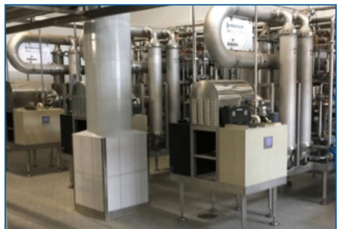
Pentair BMF System at Einbecker Brewery, Germany
