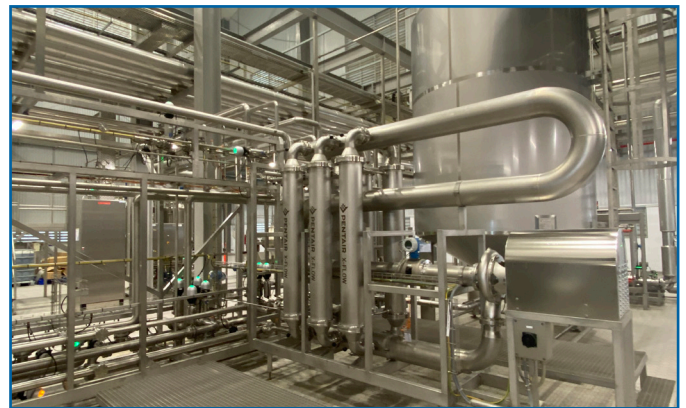
Pentair Beer Membrane Filtration System at Hanuman
